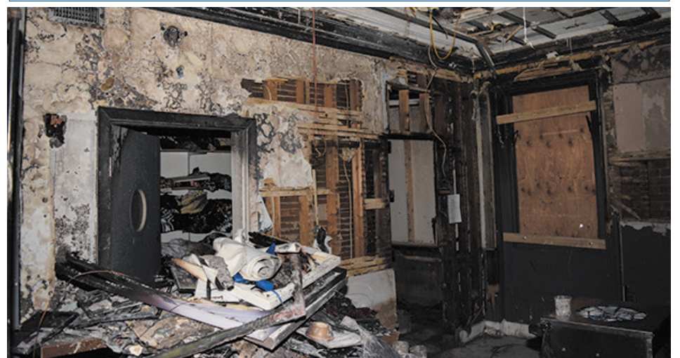
Damage from the 2016 fire that started in the second-floor art gallery in the Newbury Street building in Boston
